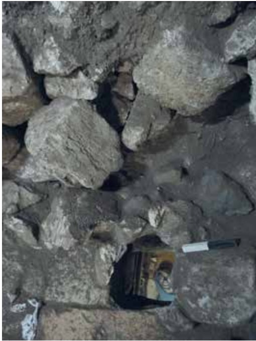
Fig. 4a. View of the manhole that connected the drainage channel to the street, during excavation.
